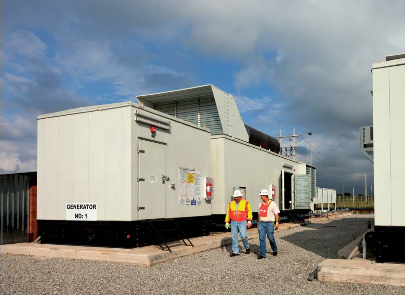
Peet du Toit and Lourens Bayliss at the back-up power generators at Anglo Platinum Limited's Khuseleka Mine.
