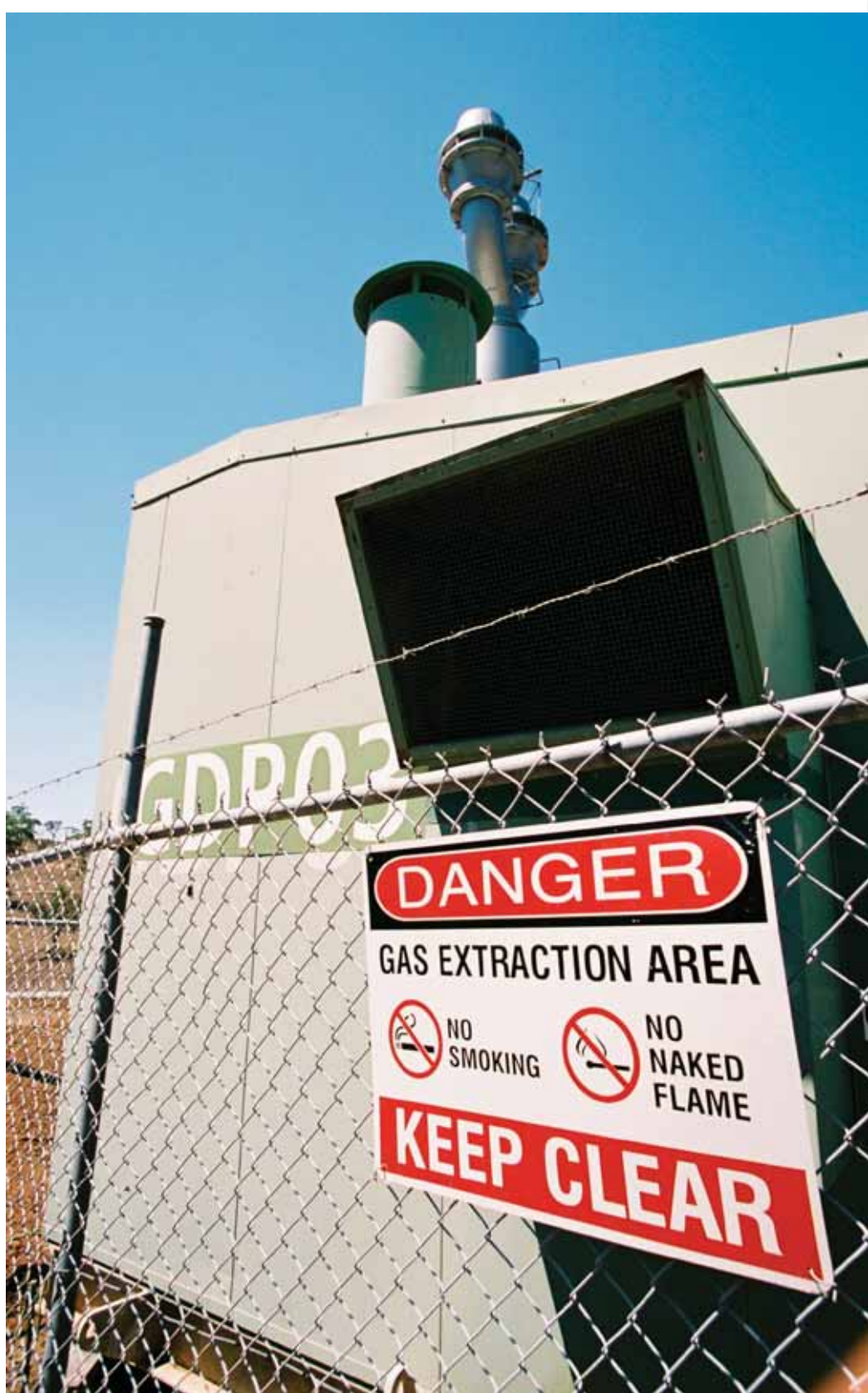
Above: Infrastructure for the methane flaring trial.
